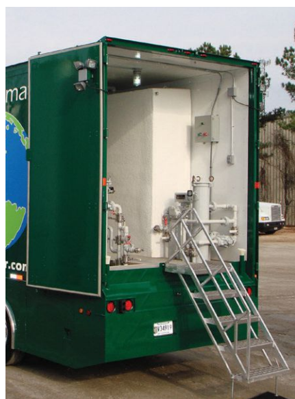
Figure 2 | A vacuum dehydrator on the truck. (Photo courtesy of Billy Byrd and John Erickson, Dilmar Fluid Services.)
